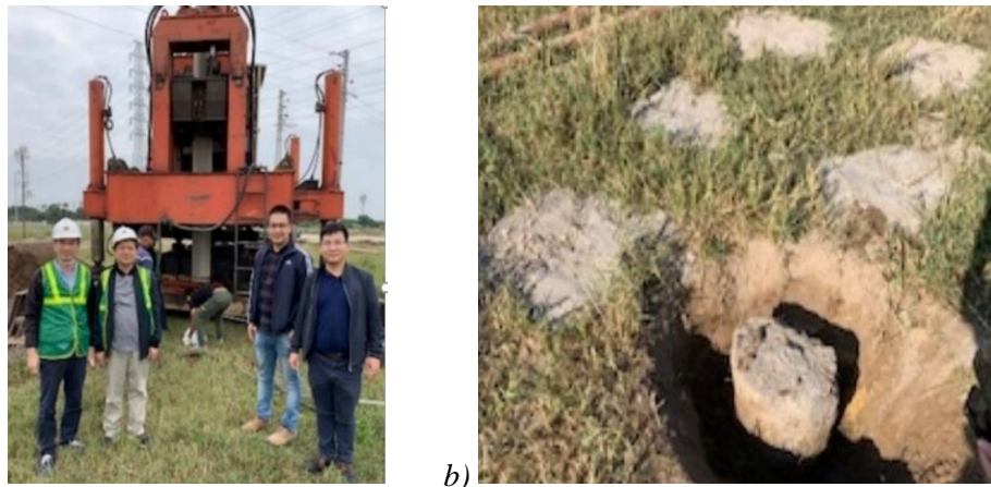
Fig. 7. a) TP300 pile pressing robot; b) CFMS pile after 10 days of construction
