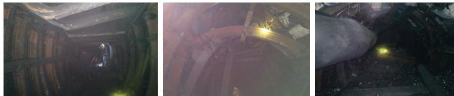
Fig. 7. Manifestations of gateroads under abutment pressure: a. Reduced cross-section, b. Broken column heat, c. Floor heave
